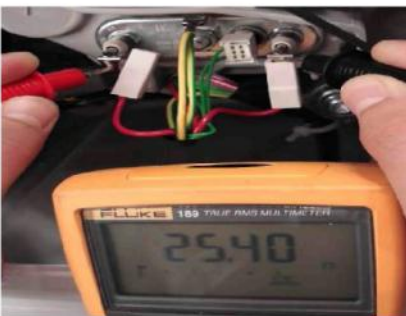
PICTURE E2-4: One of the cables (left one) on the heater has been removed and heater resistance is being measured.
