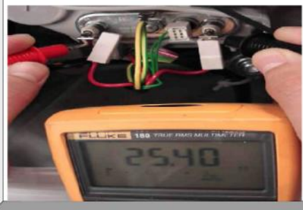
Picture E3-4: Heater Resistance measurement
