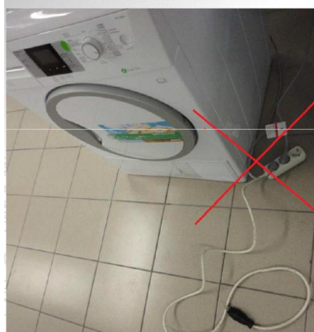
Inappropriate Extension Cable Usage
