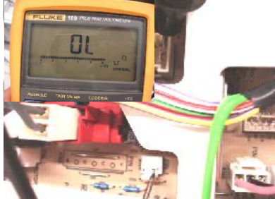
PICTURE E2-3: Short circuit check is being made between KN8-1 pin and KN5-1 pin.
