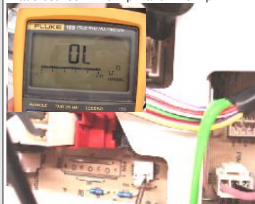
PICTURE E2-3: Short circuit check is being made between KN8-1 pin and KN5-1 pin.
