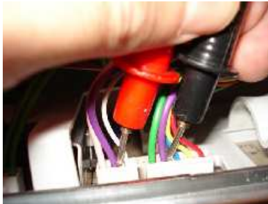
PICTURE E5-1: Voltage value going to the pump via card is being measured
